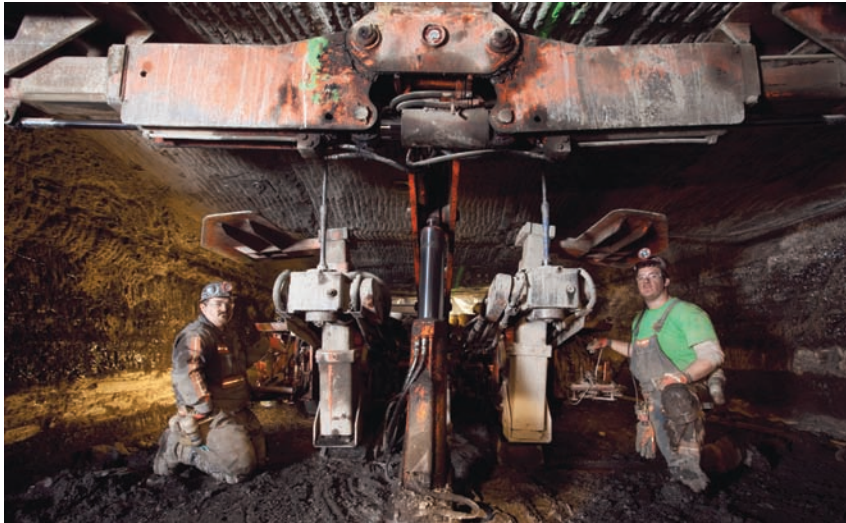
Left to right: Jasher Norman and Brandon Hatfield perform roofbolting work at Rockhouse's No. 3A Mine. Like so many in the industry, both are multi-generational miners.
